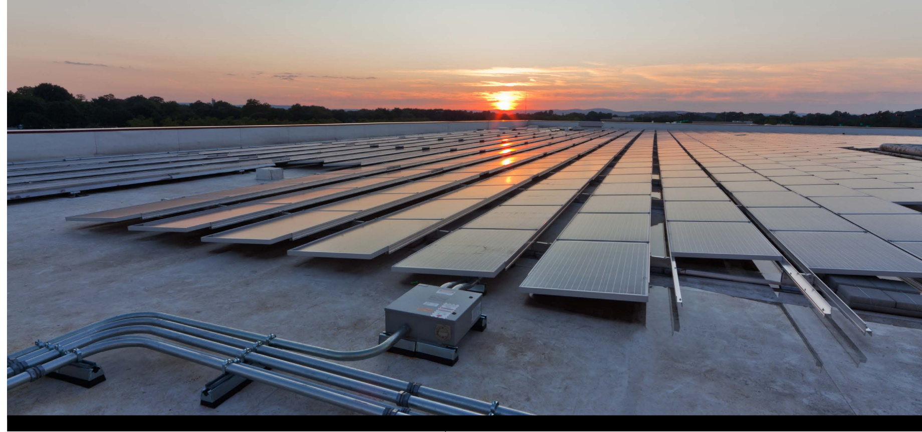
900 kW SOLAR PROJECT AT BERGEN TOWN CENTER IN PARAMUS, NJ
